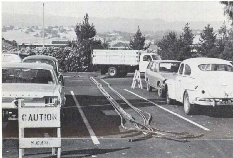
BURIED TREASURE. Just as there is "more than one way to skin a cat," there is also more than one way to make productive use of formerly useful but now unneeded materials. This was discovered during the week of July 12 when nearly 5,000 feet of 500 MCM copper electrical wire was removed from underground ducting that ran from Building 3L to the southwest property line of the Stanford plant. This cable was originally installed in 1961 as the main electrical feed to the plant, but was replaced by larger service in 1966 as Buildings 5 and 6A were added to the complex. No longer needed in its underground location and unusable elsewhere, the cable was removed by GENE FORRESTER's Technical Maintenance and DICK ELY's Building Services people at a cost of $300. It was then taken to a scrap dealer who weighed it and wrote a check payable to Hewlett-Packard for $1973.70!
